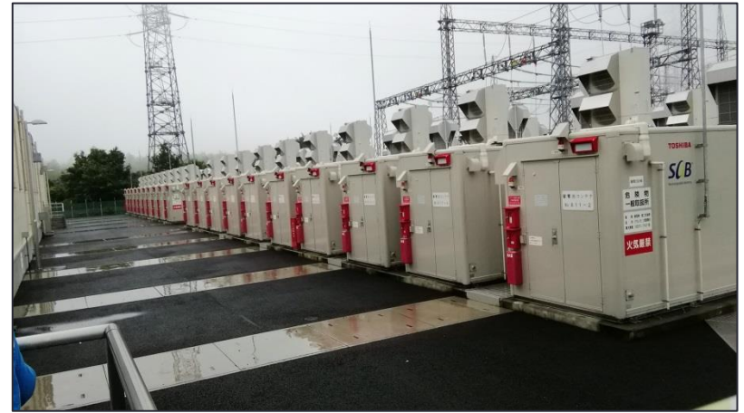
Battery arrays (Nishisendai Substation)
